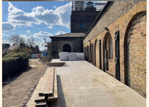
Works on the Engine House, second floor gallery and external terrace © Quentin Blake Centre for Illustration
